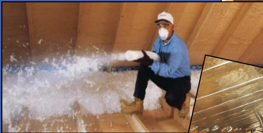
Blown-in Insulation Vented Attic
