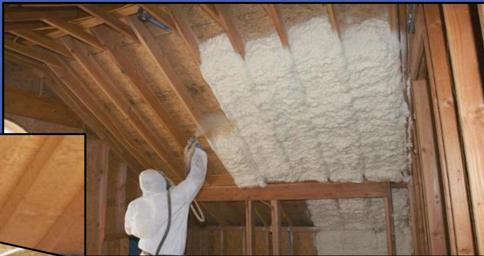
Foam Insulation Conditioned Attic
