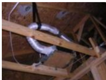
Poor installation (U bend)
